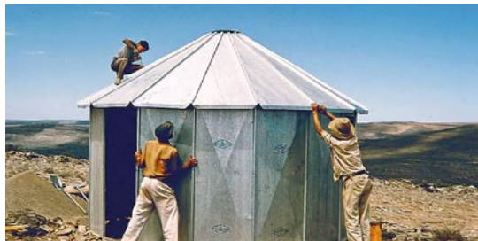
Fig. 13: Ample use was made of “rondavel”-type of temporary buildings which could easily be erected and broken down again, particularly handy in the mountainous terrain of the Nieuwveld plateau. Credit: ESO, J Doornenbal
