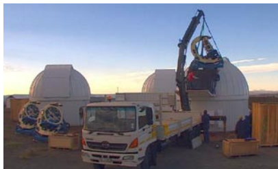
At the crack of dawn (picture taken at 07:15, to be exact), the first telescope was being installed into its dome.
